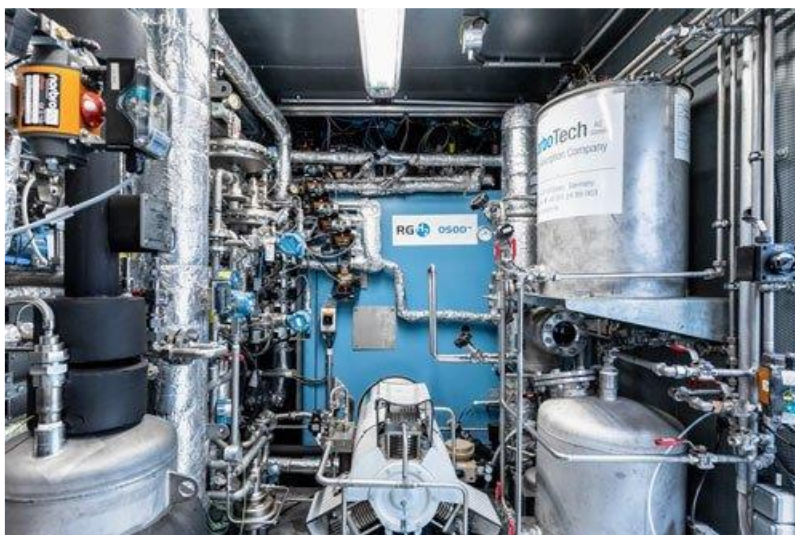
Figure 12 The inner workings of the OSOD H2 generator. The blue cuboid is the core development: a gas furnace with four tubular reactors in which the chemical looping process for hydrogen production takes place. (Image: RGH2)
